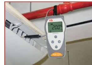
Temperature measurement in air conditioning system
